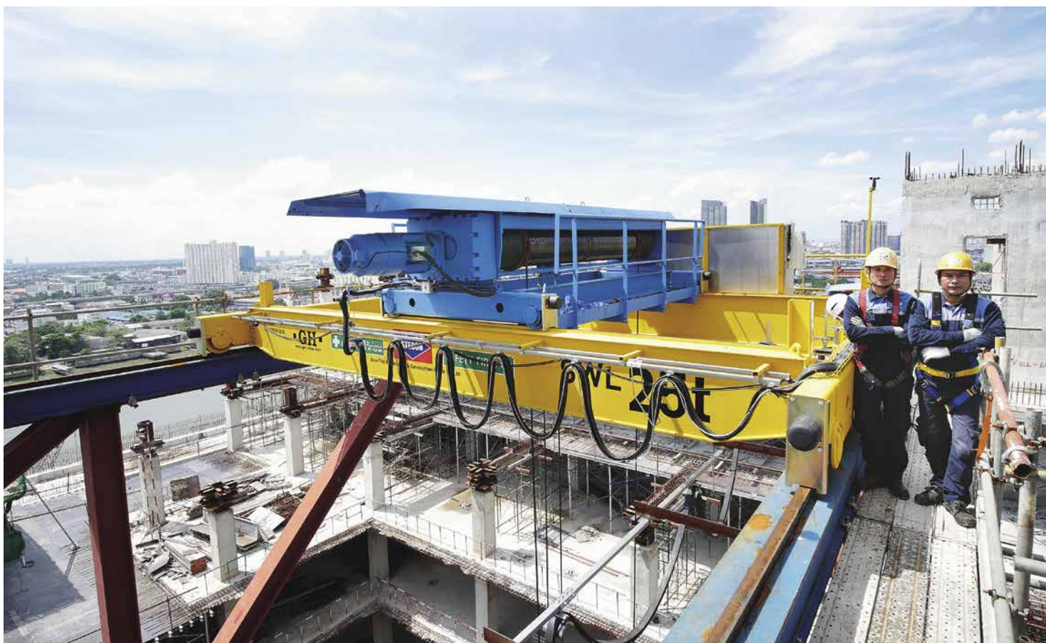
Double beam mobile crane (25t., 60m high) in a construction site that STECON operates in Thailand.
