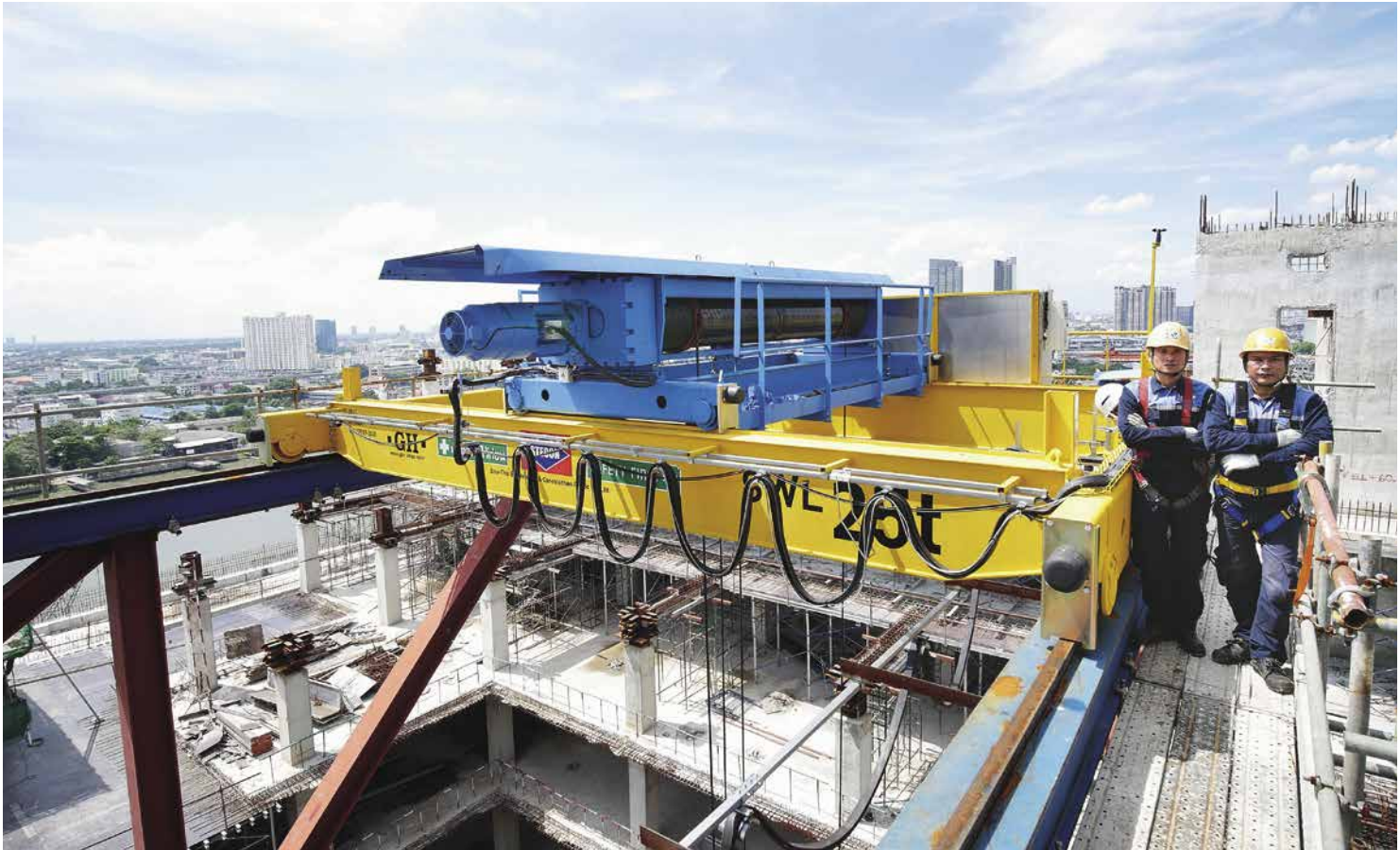
Double beam mobile crane (25t., 60m high) in a construction site that STECON operates in Thailand.
